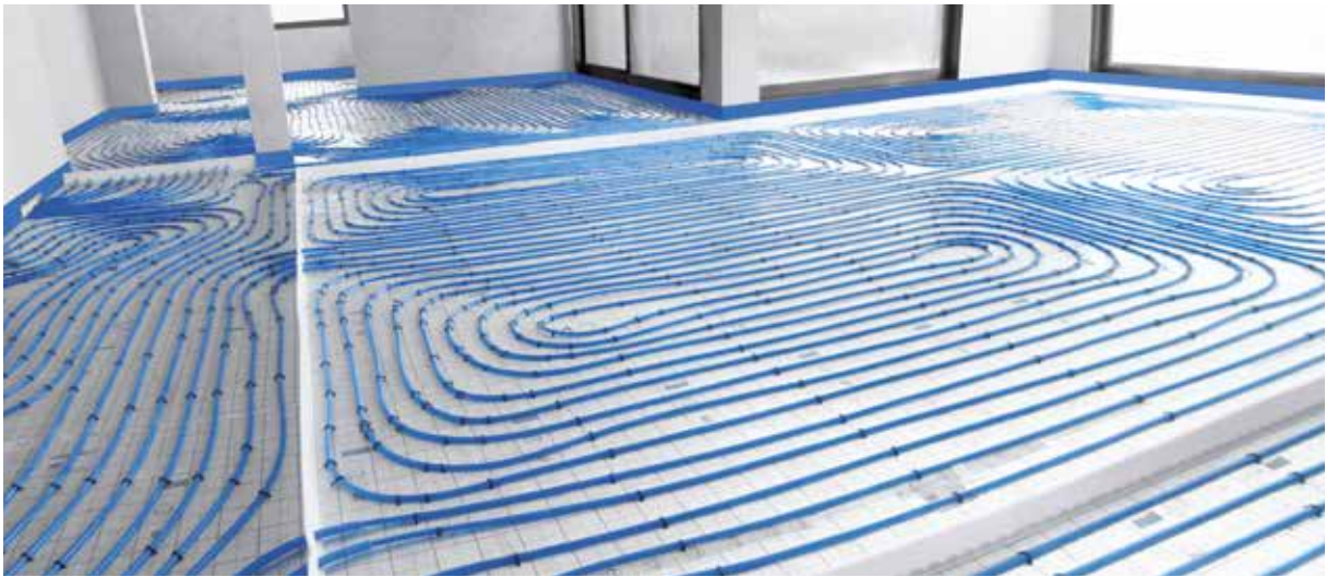
Fig. 25. KAN-therm Tacker system floor heating/cooling.
