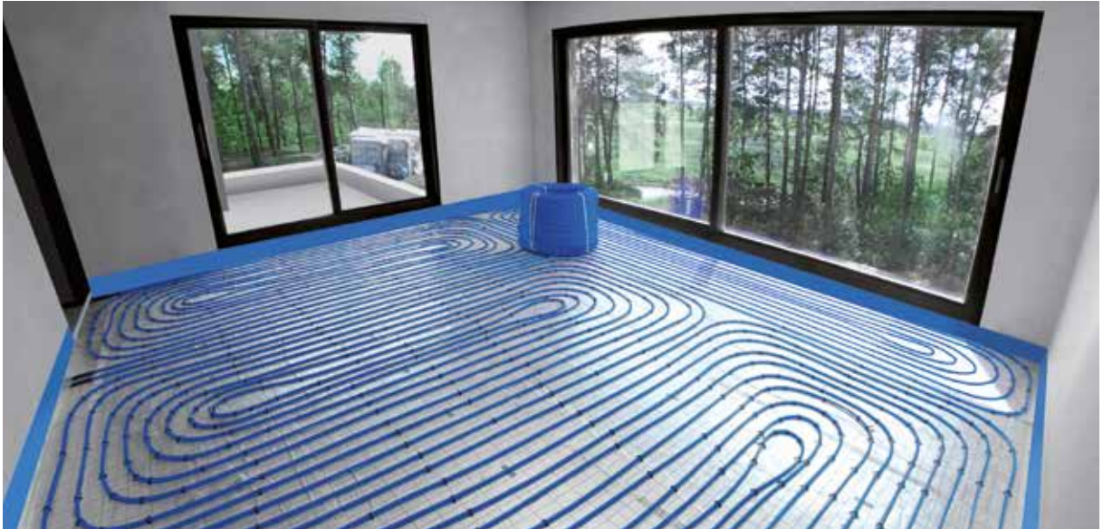
Fig. 3. Floor heating installation in single-family building, employing bluePERT pipes and KAN-therm Tacker system.
