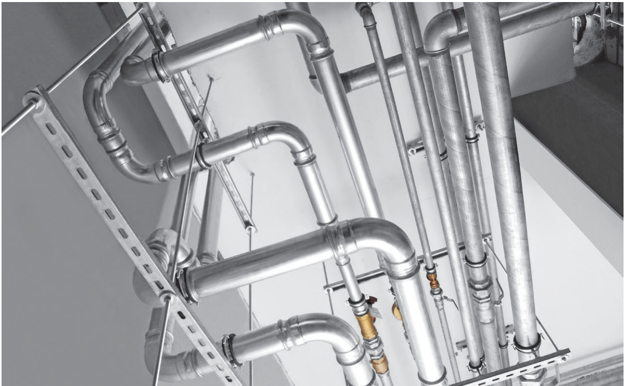
Exemplary KAN-therm Inox installation
