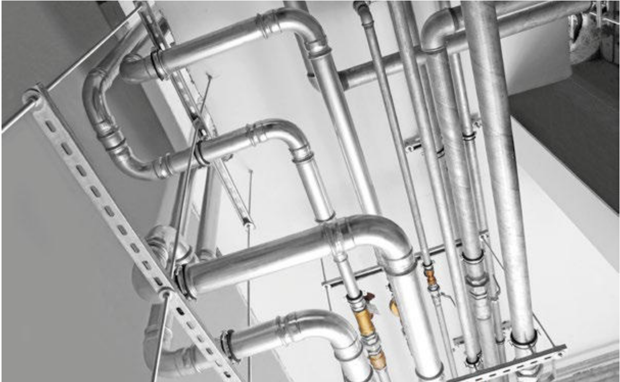
Exemplary KAN-therm Inox installation
